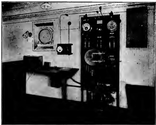
Standard 2-kw. equipment as installed.
